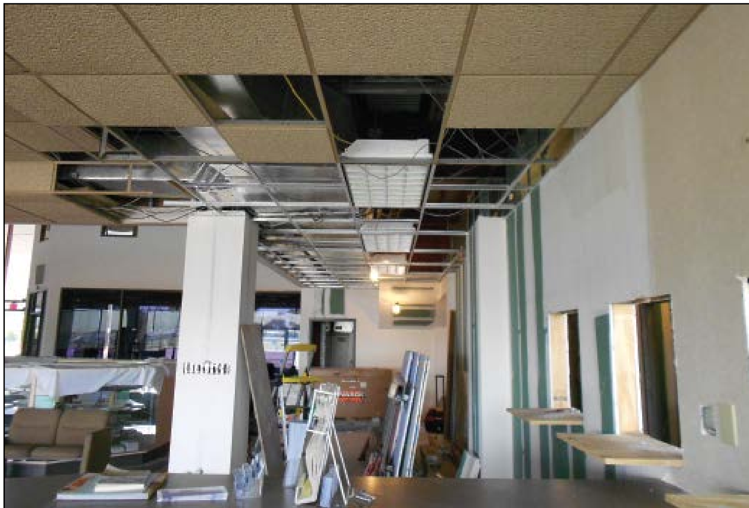
ABOVE. Recent renovations on West Houston's terminal gutted the existing building built in 1984
