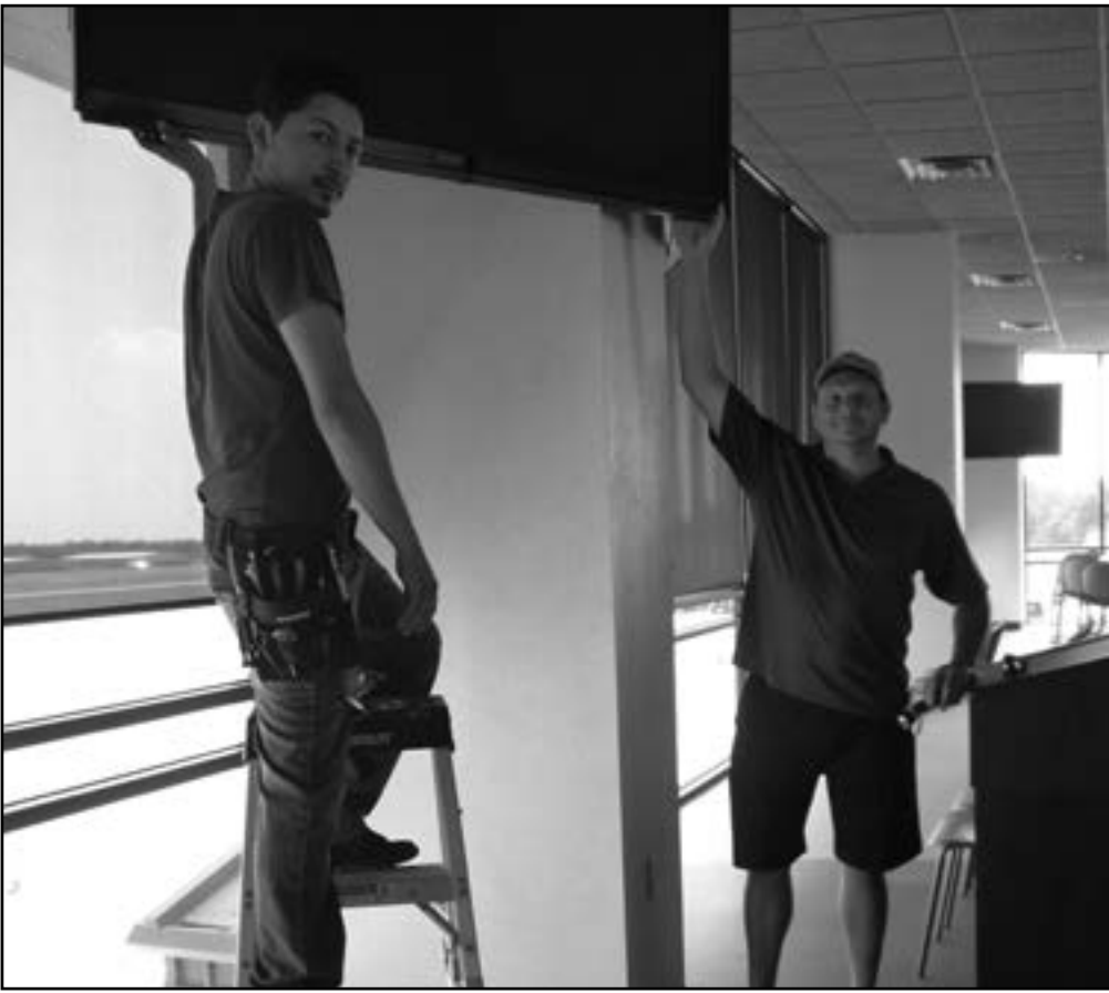
ABOVE. John Conley of ICS installs flatscreen TV at West Houston
